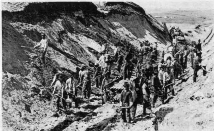
NORTHERN PACIFIC CONSTRUCTION —Grading crews, working with picks, shovels and horse-drawn wagons, are shown here constructing the NP right-of-way through Dakota Territory in 1879. Photo was taken of the Big Cut in Sweet Briar Valley. The Railway celebrates its Charter Centennial on July 2 of this year.
