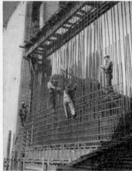
Men at work on just one spot of the mass of steel that is going into the concrete forming Grand Coulee dam in the Columbia river in Washington, man's greatest construction job which will hold back waters of the mighty river and make them available for irrigation of 1,200,000 acres.
