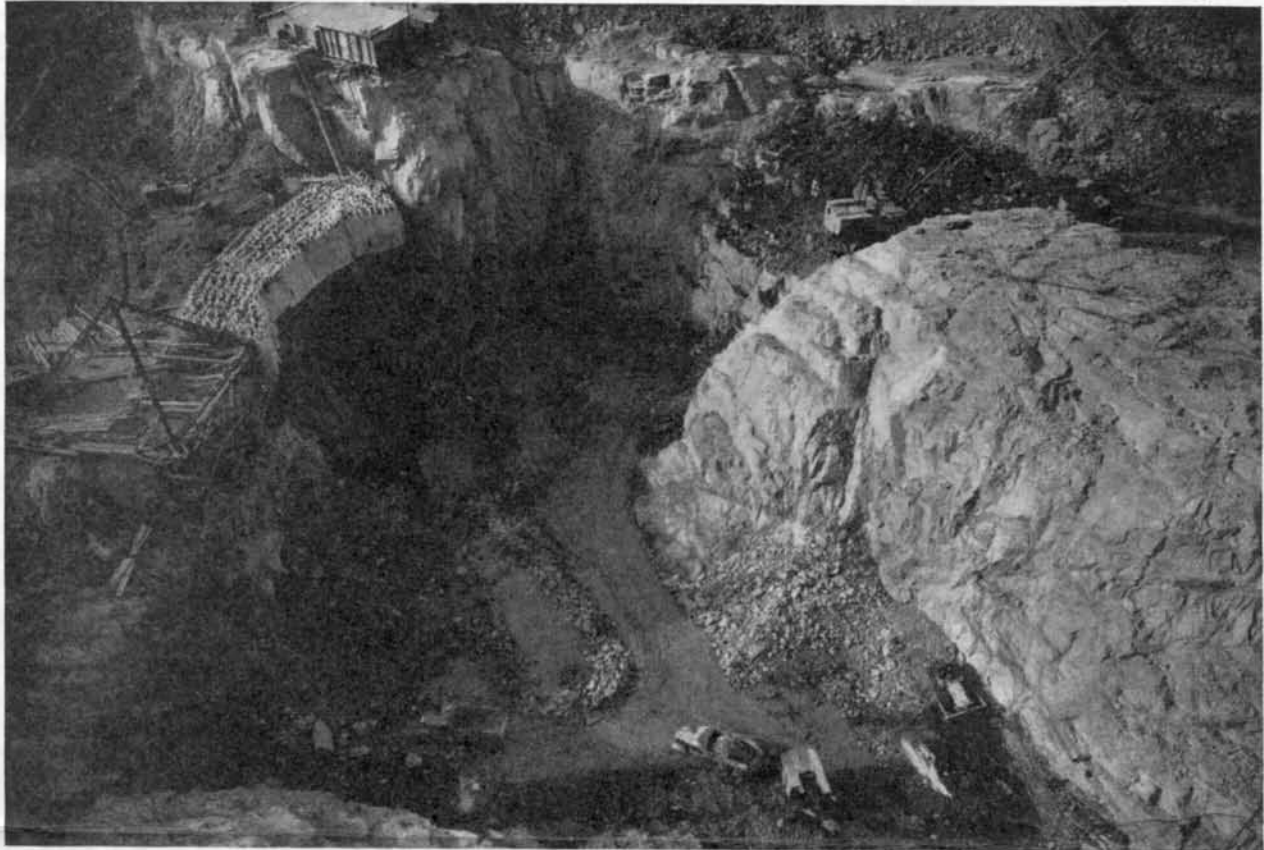
Frozen arch of earth at the site of Grand Coulee dam on the Columbia river which holds back a slide while construction is in progress. Brine pipes going down through the silt are seen at the left over the entire area of the frozen dam. The pipes are white-surfaced and curved at the top. In front is the base of crevice which the slide filled. It is now cleared out to bedrock. Thus a dam of frozen earth was effective.
