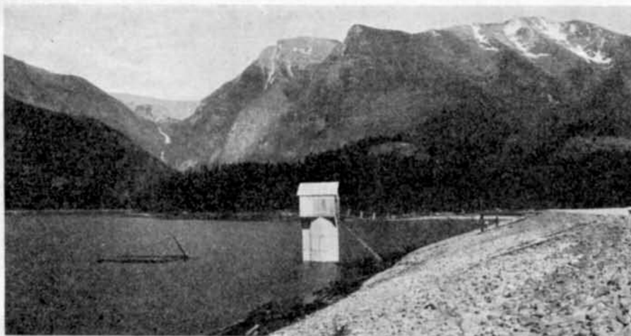
New dam in Mission canyon, Lake county, western Montana, is a part of the irrigation works on the Flathead valley project, further assurance of water for crops. Completed a few weeks ago, it is 90 feet high, nearly half a mile long and provides a reservoir for 8,000 acre feet of water. As shown here, it has 52 feet of water in it at the dam. The small house in the center is the control room for regulation of stream flow below the dam. In the background is the Mission range and at left background, a mountain falls which looks like snow. Timber cut from the reservoir site was used for project construction work, the slashings and brush being burned in the reservoir before it was flooded.
