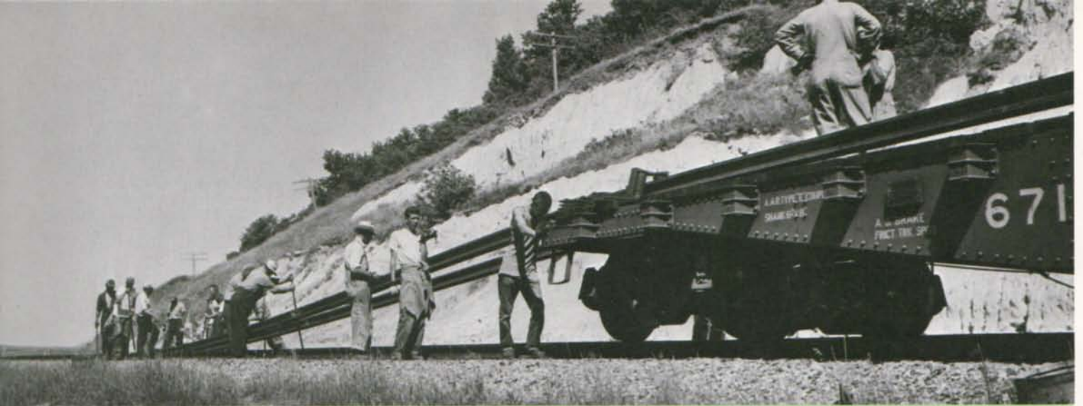
Quarter-mile-long sections of welded rail are used in Burlington Northern's main line track relay program.
